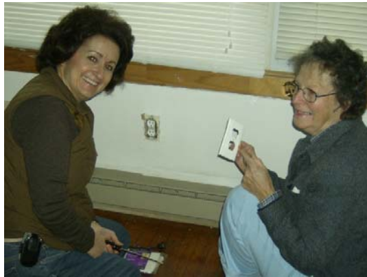
Holly Kay Prehn and Emily Daniels insulate the electrical outlets and light switch plate fixtures to help minimize cold air from coming in and the heat from going out. You can get tips and recommendations on how to make your home energy efficient by visiting www.agingtogether.org and clicking on AARP's Operation Energy Save link.
